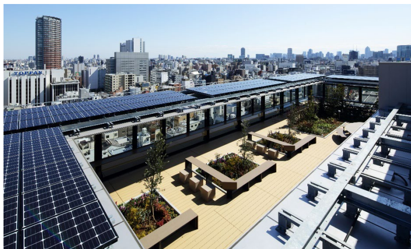
Solar panels installed on the roof of Head Office
